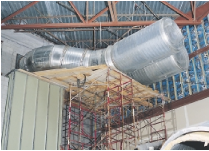
Duct Silencers, The First Assembly of God—Grand Rapids, Michigan
