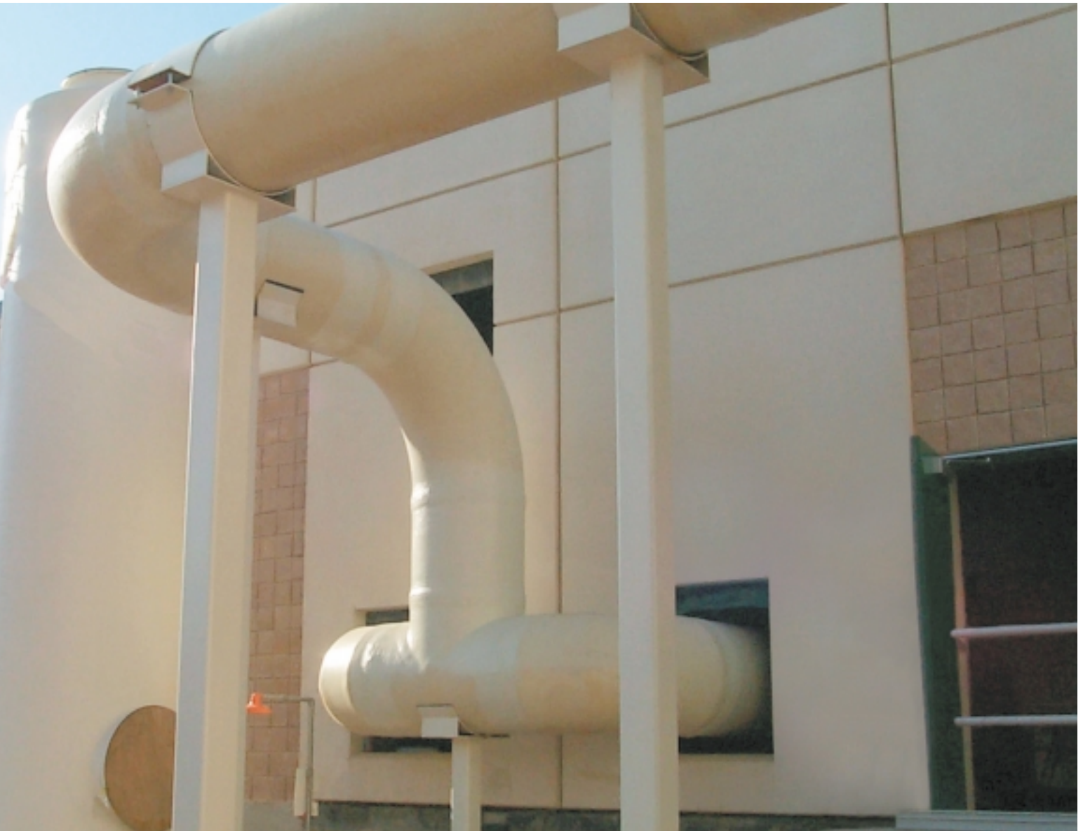
FIBER-PLAS ductwork, Gwinnette Waste Water Treatment Plant—Gwinnette, Georgia
