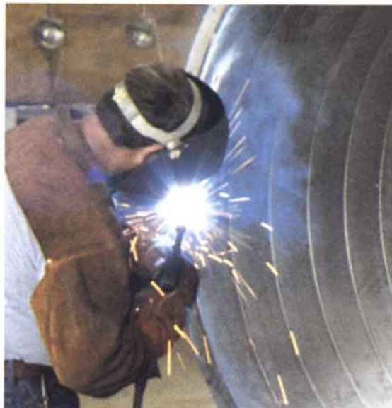
Flanges were welded to the sections of duct produced by the mobile duct machine.
